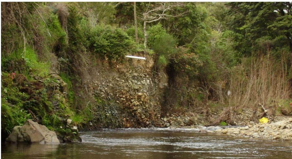
■ Figure 2 Erosion Hazard Identified Adjacent to Maymorn Road, Areas B and C
