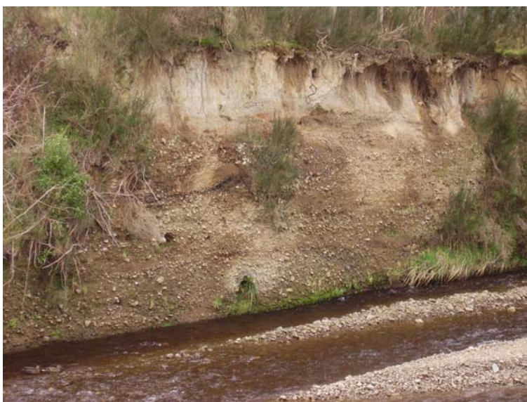
■ Figure 5 Mangaroa Hill Bridge Erosion Area
